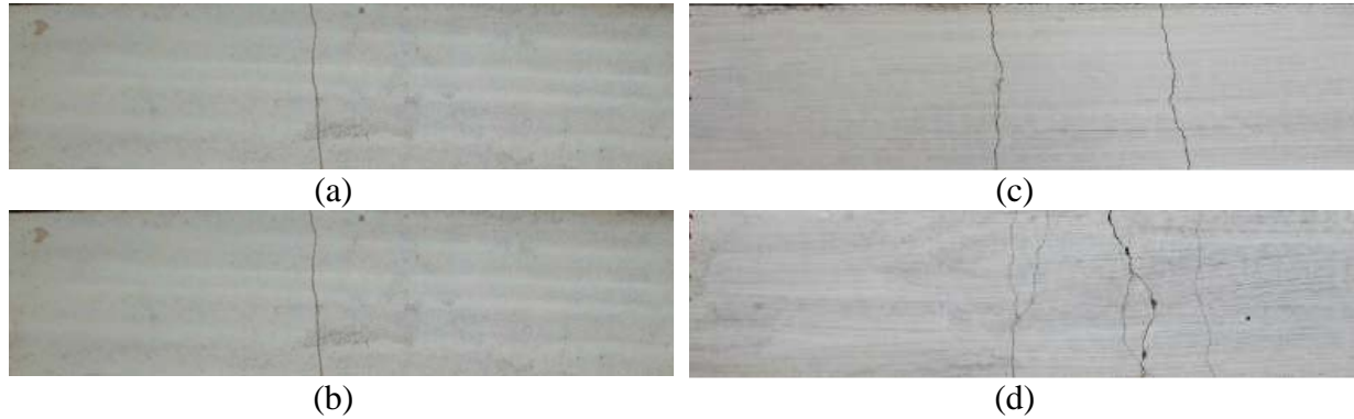
Figure 5. Typical cracking patterns for the composites (a) R2%_25, (b) R4%_25, (c) and (d) R6%_25.
