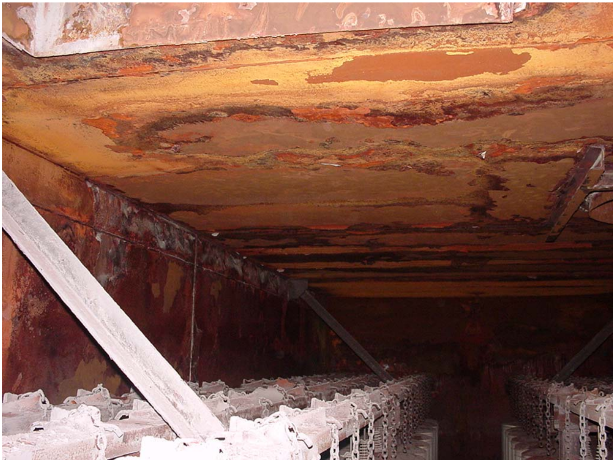
Figure 1. Severe corrosion damage in a reverse air bag house filter.
