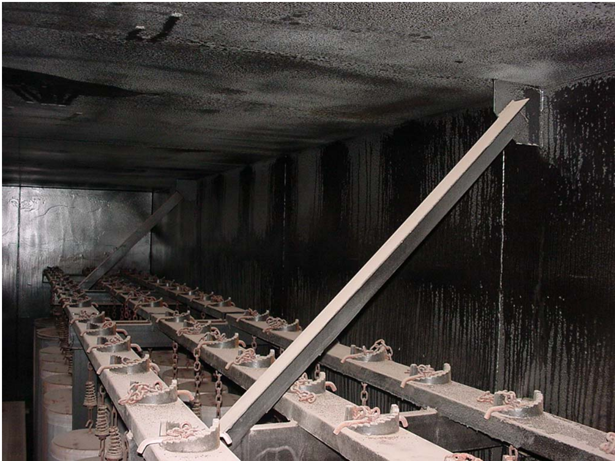
Figure 3. Inspection of FlueGard-225 after 2 years in a bag house filter. No corrosion.
