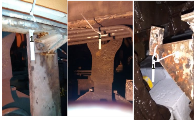
Figure 10. (1) – corrosion samples installed in exhaust chamber to evaluate the corrosion rate
