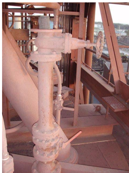
Figure 8: Deflector grill at reduction furnace discharge.
