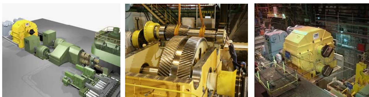
Figure 5. New drive behind existing drive unit (drawing, left), installation of gear unit (middle), shifting of foundation block (right).
