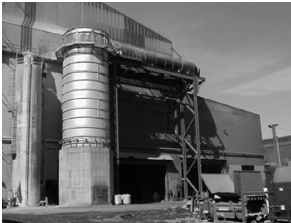
Figure 7. A spray tower installation for quenching DEC gas.
