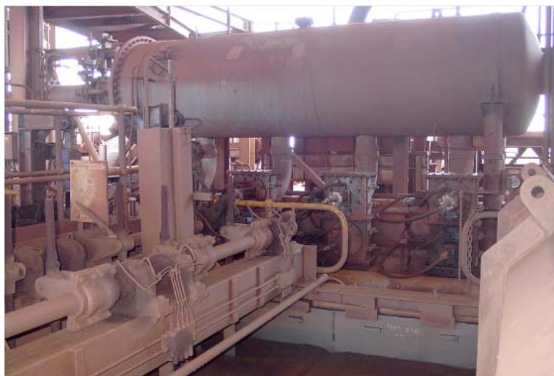
Figure 3: Iron ore jigs, Port Headland plant
