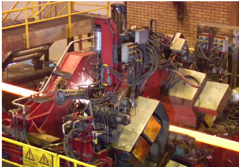
Figure 02 Welding unit of ERT-EBROS
