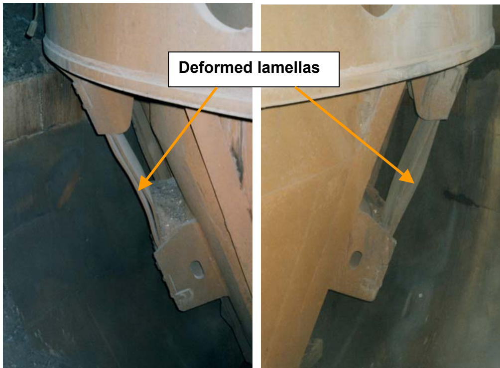
Figure 1: Converter Before Exchange in 2003
