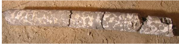
Figure 6 Core taken out of drilled hole; presence of coke will contribute to the recovery
