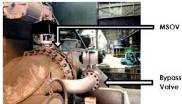
Figure 2: Bypass valve installed parallel to the MSOV
