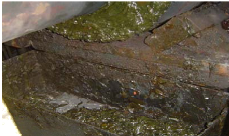
Figure 14. NSBS Grease Catch Pan.
