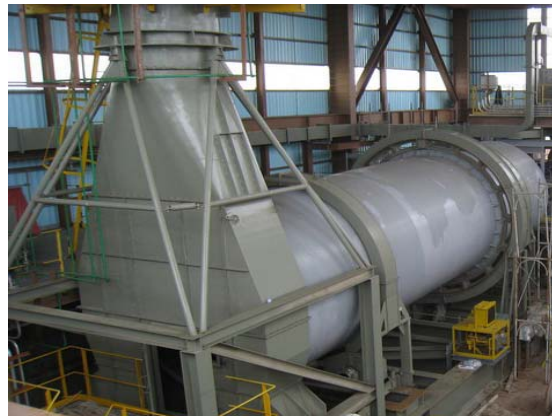
Figura 7. Horizontal granulation drum at the sinter plant no.1, Dragon Steel Corporation
