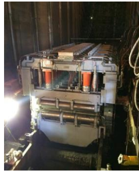
Figure 14. Installation of two SRD Segments on strand 1 of CCM1 at position 9 and 10.
