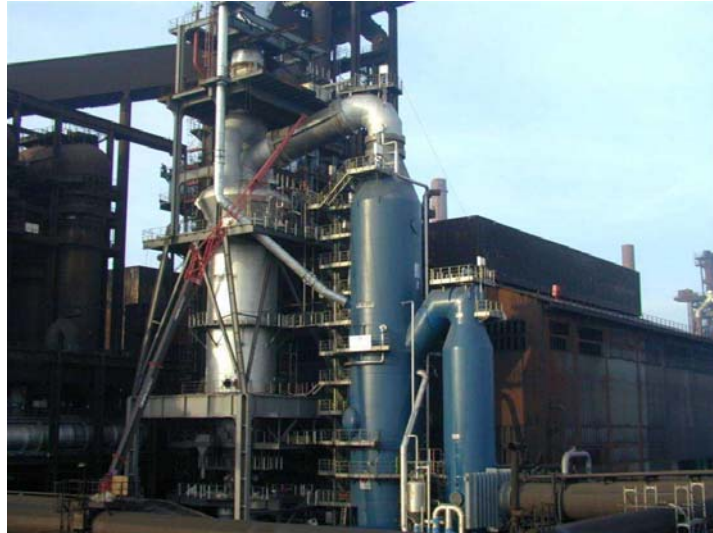
Figure 4. Gas cleaning plant ArcelorMittal, Bremen BF 2, 1999.
