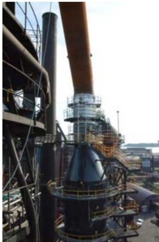
Figure 7. Gas cleaning plant SSAB, Oxelösund, BF 4, Sweden, 2012.
