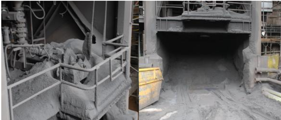
Figure 4 – Discharge area before the new BF-A gas cleaning system start-up
