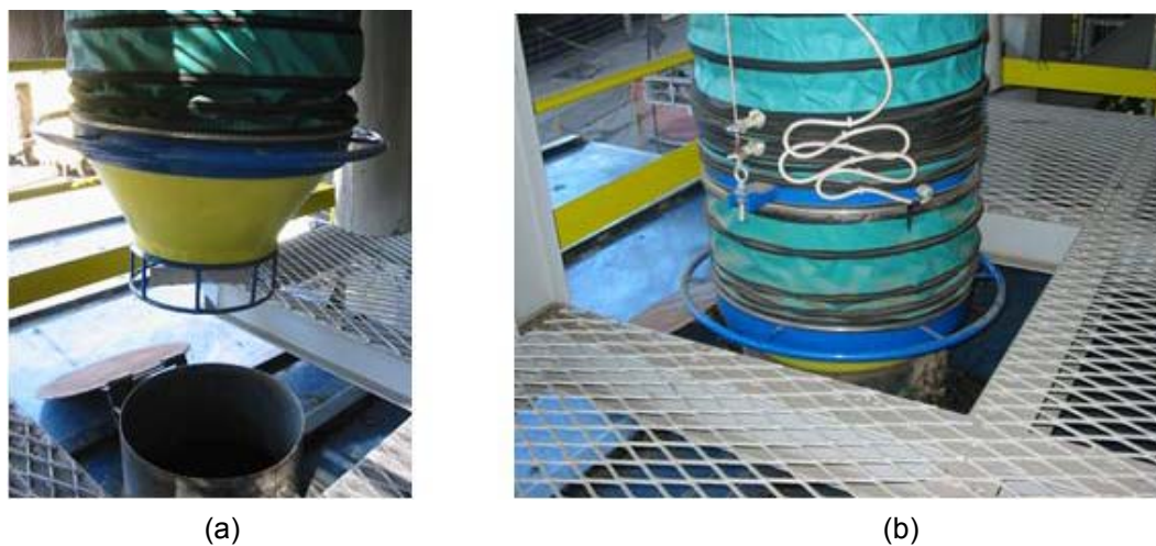
Figure 6 – Telescopic loading bellows of the dust handling system; (a) the telescopic loading bellows starting the descent procedure; (b) the telescopic loading bellows in the discharging position.
