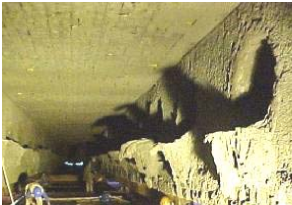
Figure 1 – Slag deposition in chamber bottom at campaign finish.
