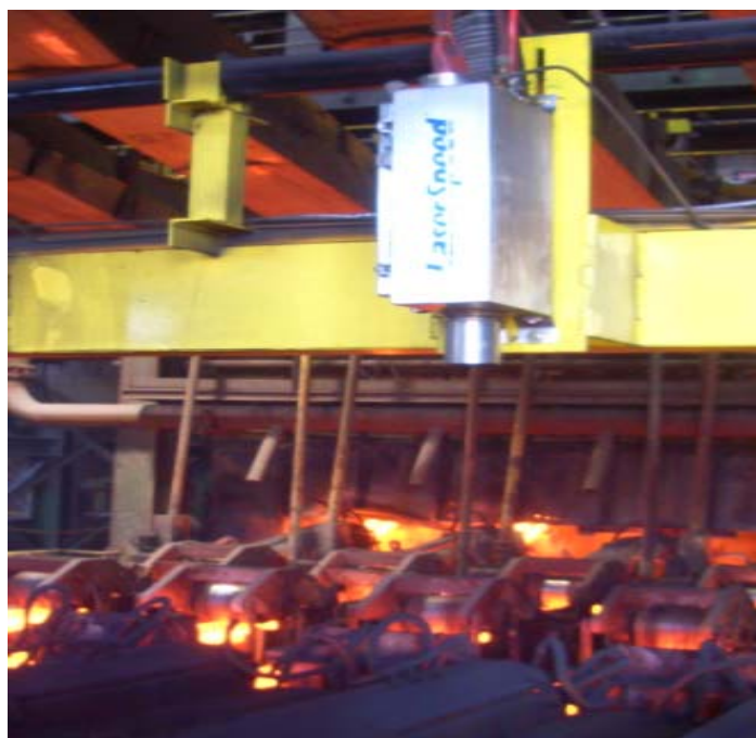
Figure 3. LaserSpeed gauge installed on a billet caster.
