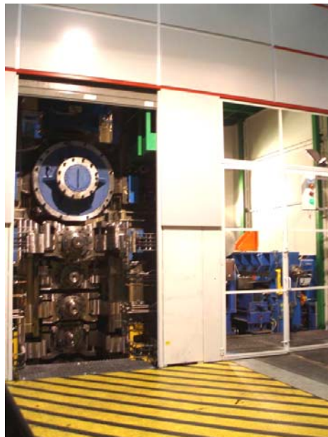
Figure 16: Tandem cold mill – mill window
