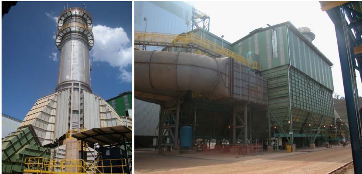
Figure 7. VSB Fume dedusting system.
