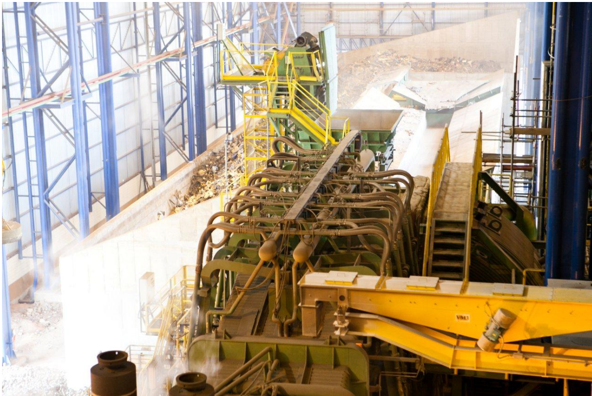
Figure 3. VSB Consteel® scrap yard.
