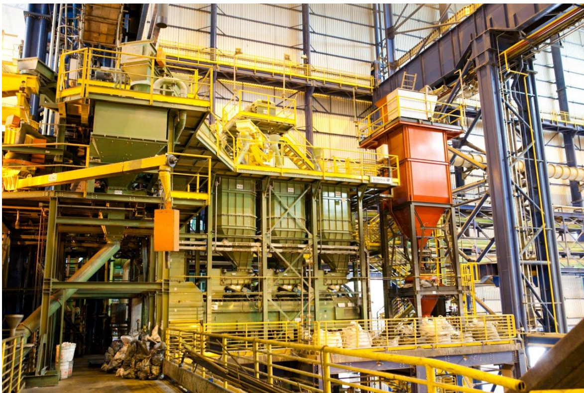
Figure 6. VSB Ferroalloy handling system.
