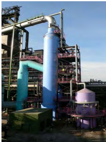
Figure 8. BF Gas scrubber at ThyssenKrupp's BF No.8.
