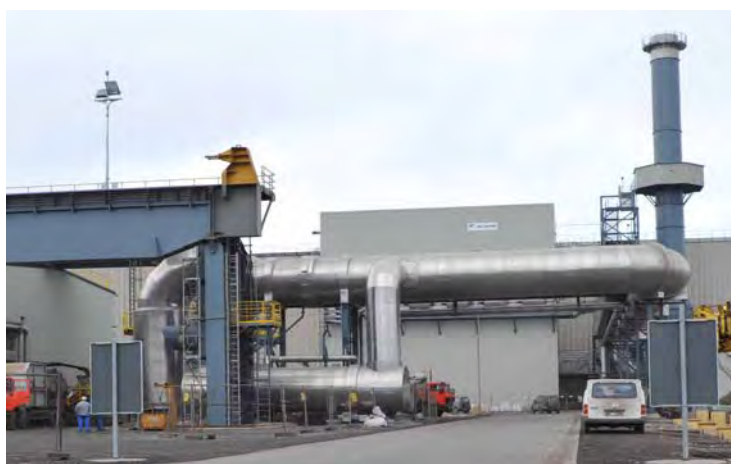
Figure 5. Heat transformer (front, middle-left) and the bag filter including chimney in the back of the picture, at the Dillinger Hütte, Dillingen Germany
