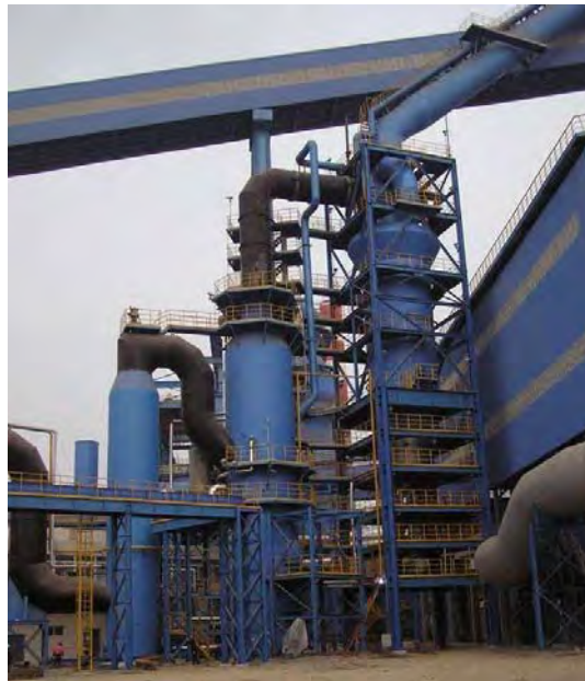
Figure 6. BF gas cleaning plant (axial cyclone, AG scrubber, mist eliminator of BF2, Tianjin, PR of China).
