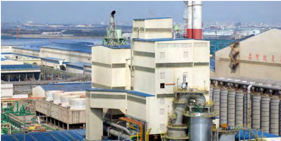
Figure 14. Primus ® plant at Dragon Steel.
