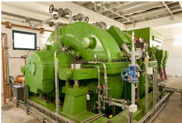
Figure 10. TRT at ThyssenKrupp Steel, Duisburg, Hamborn, BF8.
