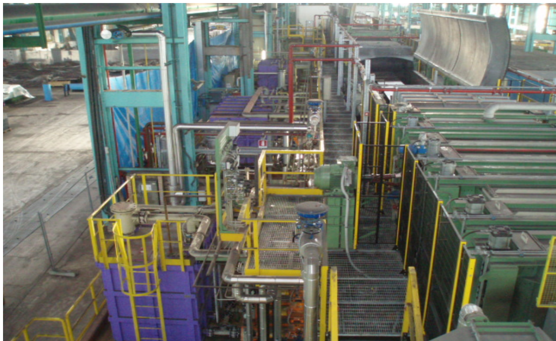
Figure 7. Pickling section overview
