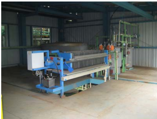
Figure 16. Silica Removal Plant
