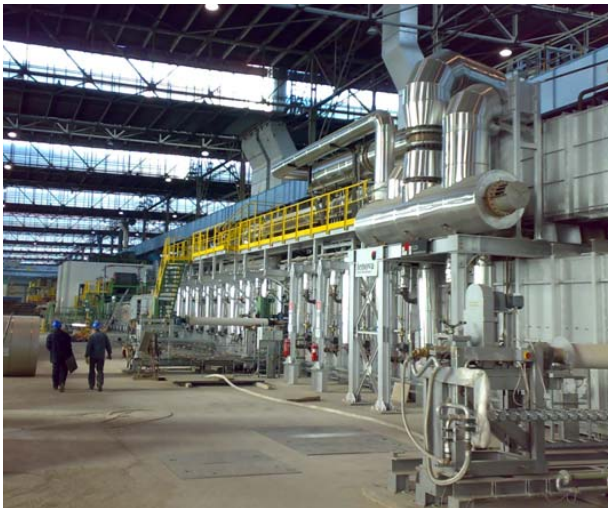
Figure 4. Furnace and cooling section
