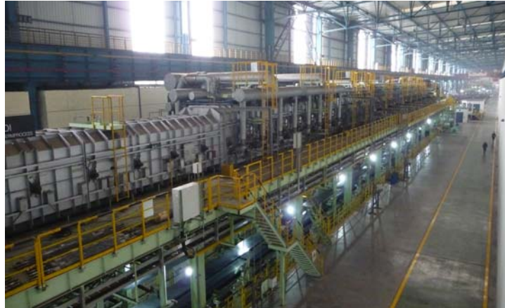
Figure 10. Radiant cooling & soaking section
