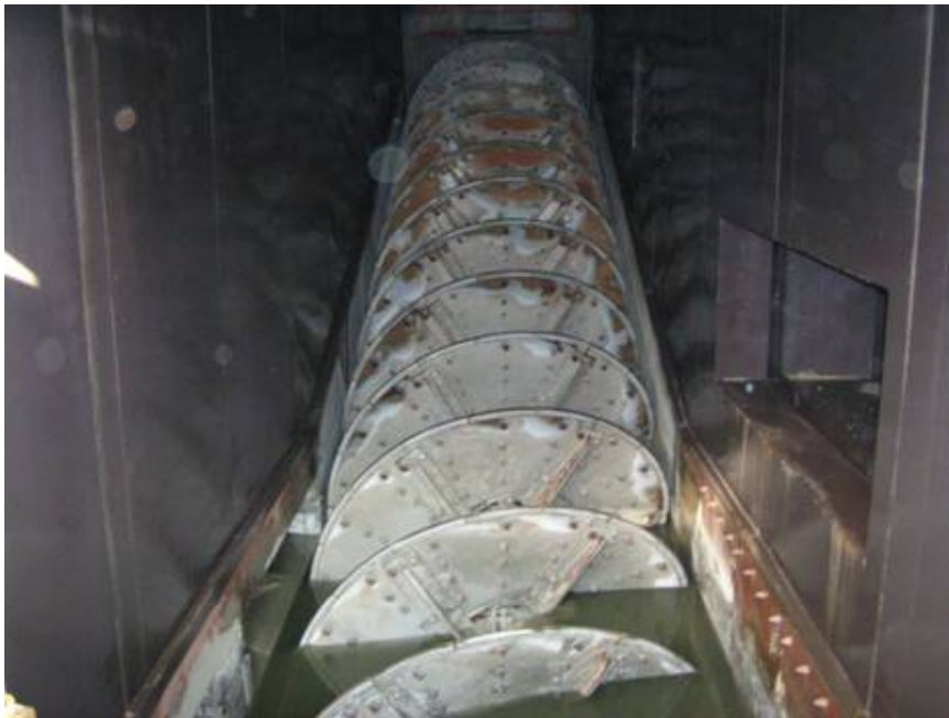
Figure 3. RASA Slag Granulation – Screw Conveyor
