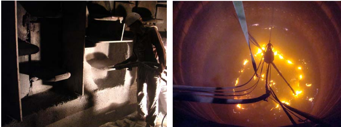
Figure 2. Cold manual jetcasting from working platform (left) and hot robotic jetcasting (right).
