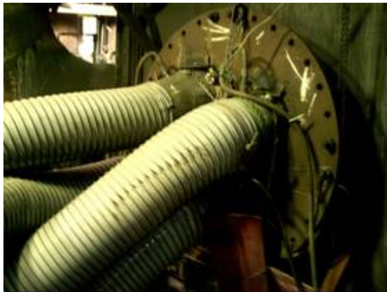
a) Ventilation System
