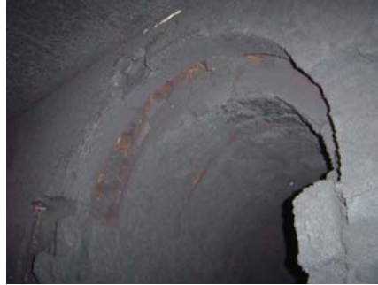
Figure 8 - Falling off of the chamber's refractory lining
