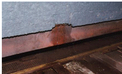
Figure 16 - Leak from a longitudinal water tank
