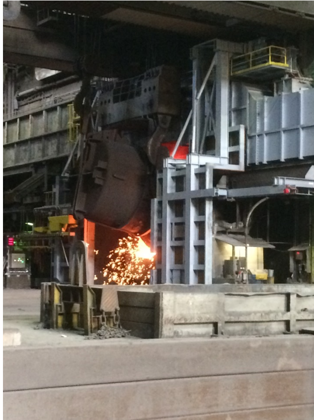
Figure 6: LD (BOF) converter supplied by Primetals Technologies at the Hochfeld works of AM.
