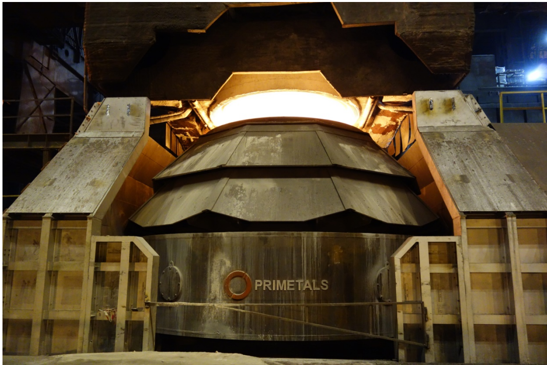
Figure 7: 315t LD (BOF) converter supplied by Primetals Technologies at AM Dabrova Gornica.
