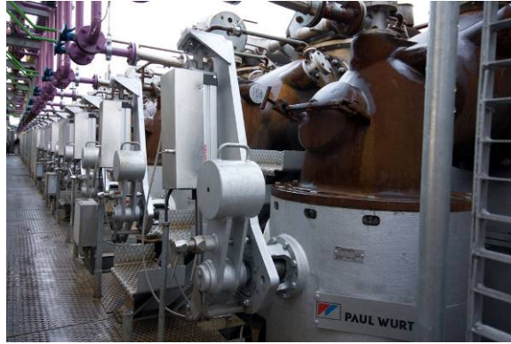
Figure 9. 50 Sopreco valves in the new Battery N° 3 of ZKS.
