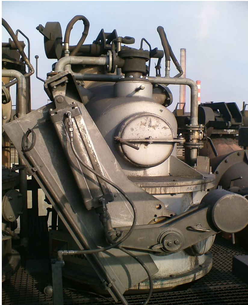
Figure 8. Realization of a Sopreco unit in the existing Battery N° 2 of ZKS.
