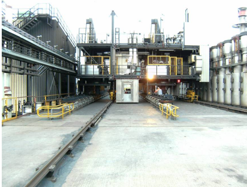
Figure 4. Service machine with a bypass gas system.
