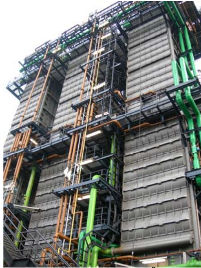
Figure 8. Primary coolers for 42500 Nm 3 /h coke oven gas each.
