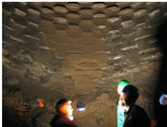
Figure 6. Example of a plate cooled bosh, demonstrating very limited wear after ten years in operation.
