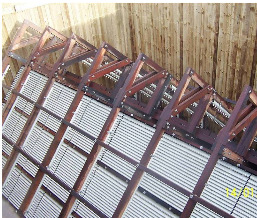
Figure 1. LEQT baffle system and flushing liquor cleaning system.
