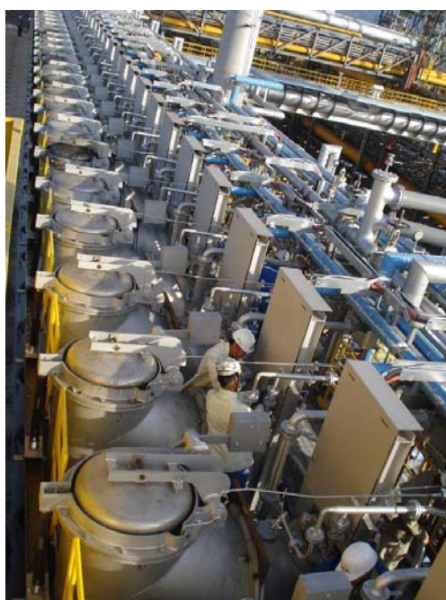
Figure 9. Space Conditions in Standpipe/Gas Collecting Main Area with a “Normal“ PROven-Equipment at a High-Capacity Coke Oven Battery.
