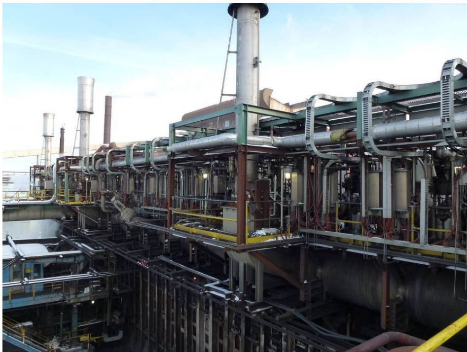
Figure 11. New Mini-PROven Installation at the Pre-Existing Coke Oven Battery No. 9 at Essar-Algoma in Canada.
