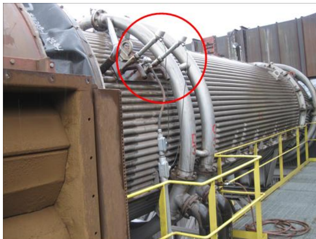
Figure 6. Outside view of the SAM sensor in the off-gas duct - simple modification and application.
