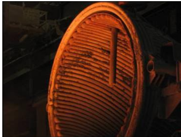
Figure 4. Lomas probe retrofit in the off-gas duct.
