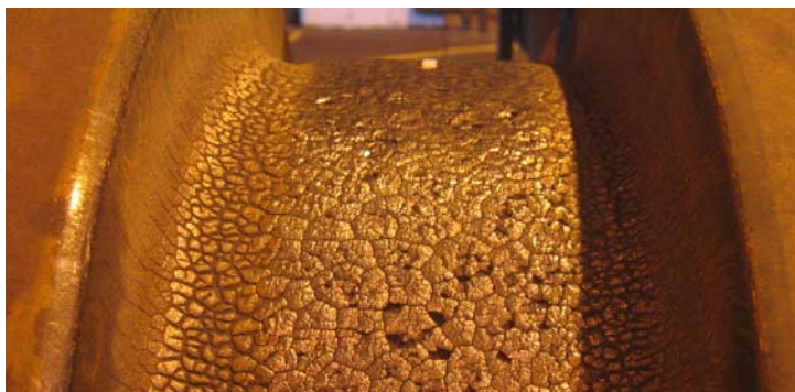
Figure 4. Severe fire cracks in a billet mill.
