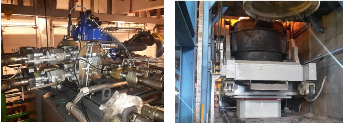
Figure 2 Hydraulic block distributors and ladle lifting table
