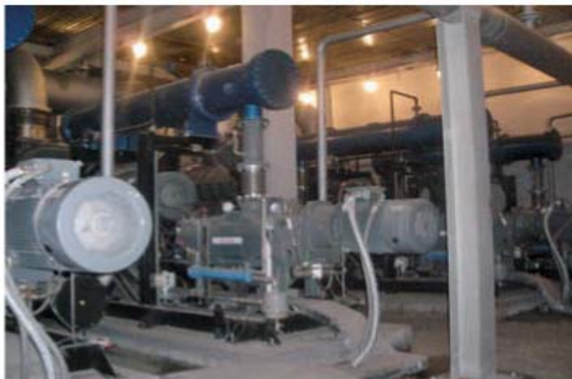
Figure 3. Four parallel vacuum pump skids in the pump room at KamaStal.
