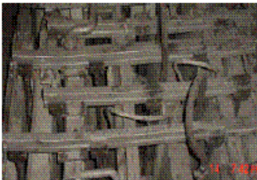
Fig . 10: Square pipe headers carrying Master Cooler SMART type air mist nozzles at HKM/Germany SMS-Demag 2-strand slab caster
