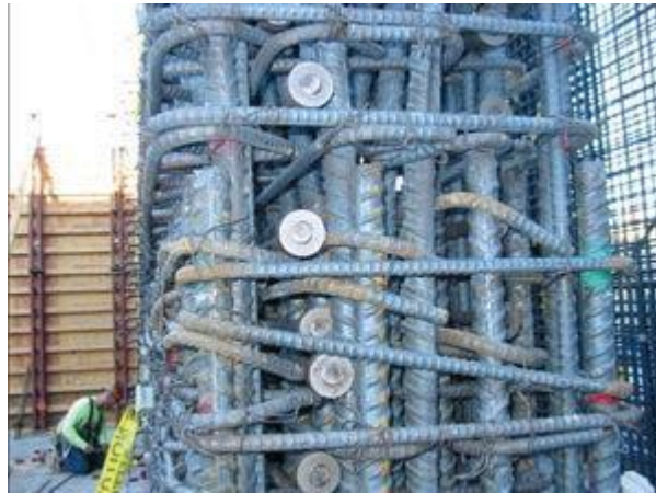
Figure 2. Rebar congestion on beam / column crossings in a high-rise building of a seismic zone (Southern California, USA).
