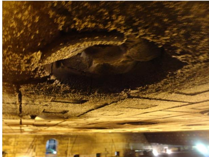
Figure 4: Visual aspect of a severely damaged refractory burner block on the Reheating Furnace's roof after 1 year operating.
