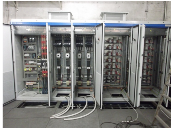
Figure 5. LV Switchboards and PLC Switchboards.
