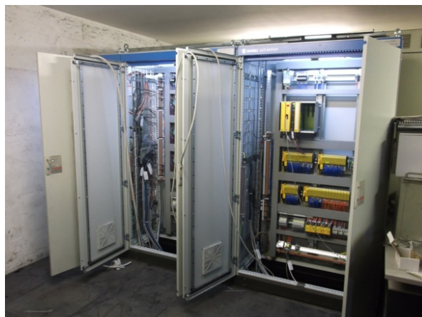
Figure 6. LV Switchboards and PLC Switchboards.
