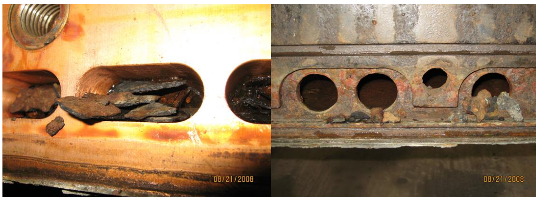
Figure 5: Scale blockage in connecting holes of a high speed copper and Scale in water jacket water feed ports
