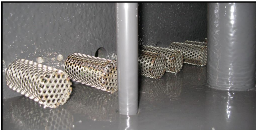
Figure 8: Bottom plenum of CSP® water jacket showing powder coating and strainers
