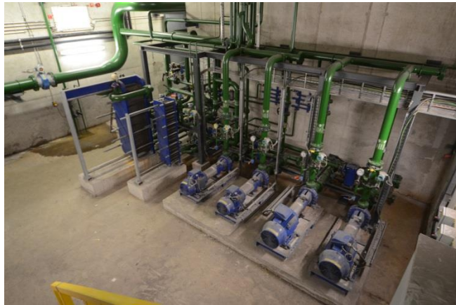
Figure 8 – Vacuum pump water cooling station
