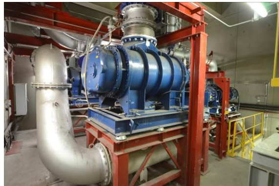
Figure 5 – Vacuum pump stages 1 and 2 with inter-stage cooling and redundancy connection
