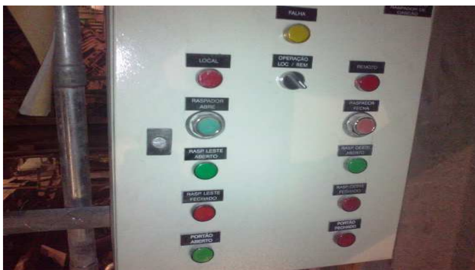
Figura 9 – Painel de controle local (RCE)
