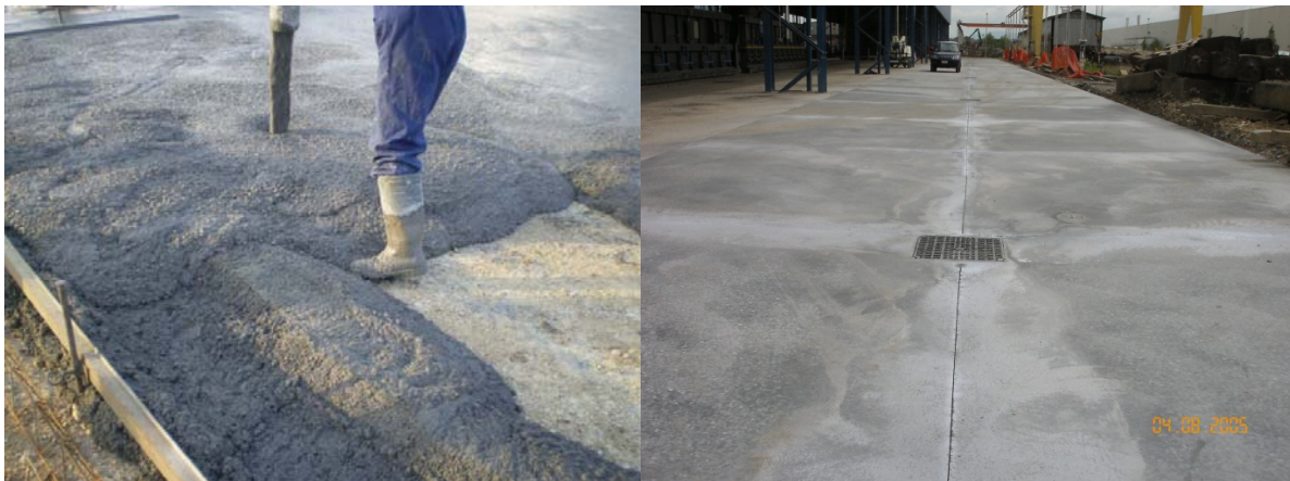
Figure 12. Concrete produced with Ecogravel like aggregate inside; and industrial concrete floor made in concrete with Ecogravel.
