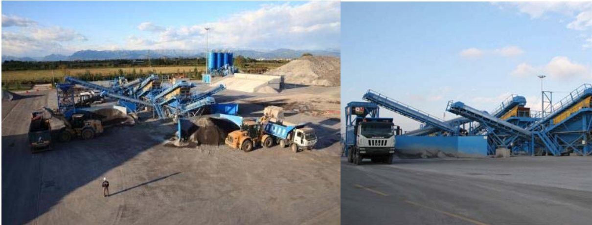
Figure 7. Danieli slag recovery plant in A.B.S. Italy; and detail of slag recovery plant.
