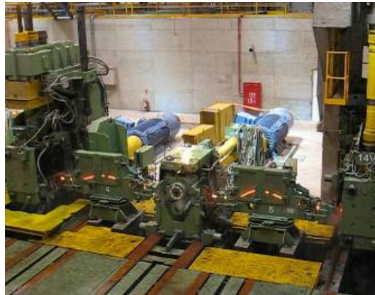
Figure 4: Finishing mill in operation.
