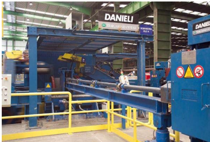
Figure 3: A spooler unit installed at Celsa Barcelona plant - Spain
