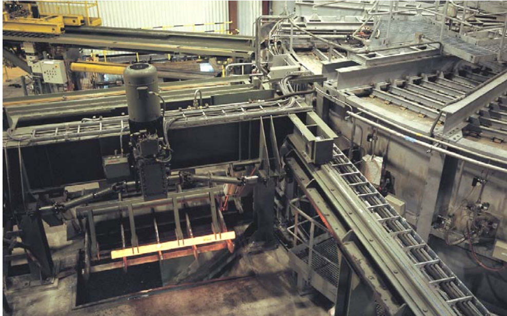
Figure 7. Rotary hearth furnace at Ovako in Hofors. Here billets for tube rolling is heated with oxyfuel to a temperature of 1200°C. The heating properties of oxyfuel minimizes the temperature deviation of max 5°C, necessary for a good piercing operation.
