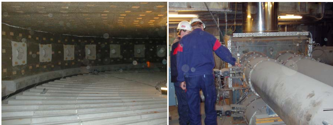
Figure 5. In the rotary hearth furnaces the heating zones and burner positions were reviewed to achieve optimum heating conditions. Refractory was not altered. Picture to the right shows the flue gas channels of 8 pit furnaces with individual pressure control exiting via one common stack.
