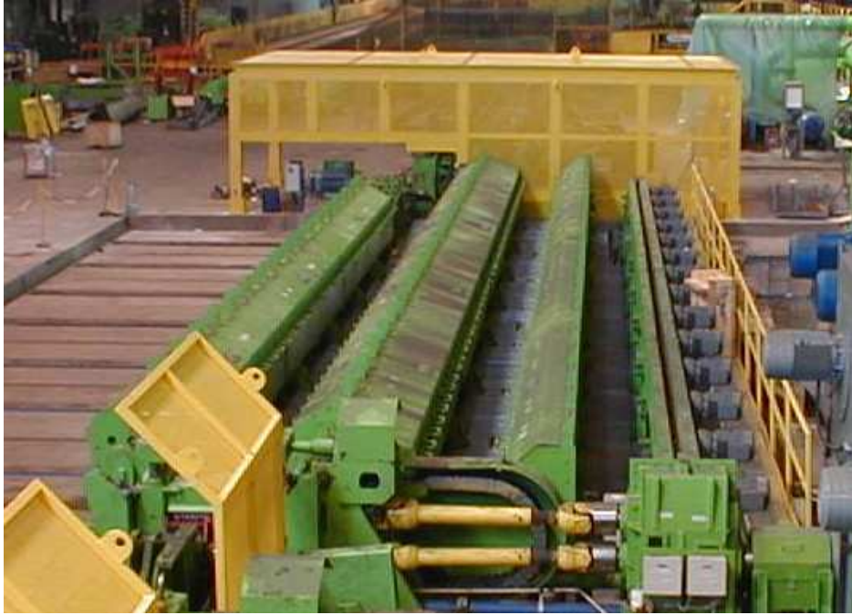
Figure 8 - Traversing water boxes for slit and single strand rolling.
