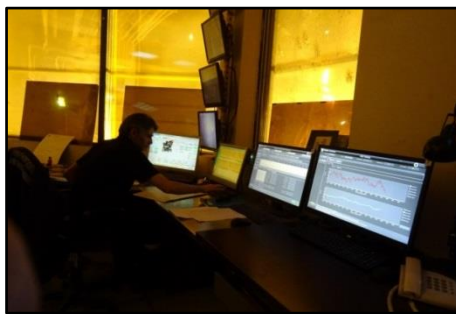
Figure 22. Control room with Q-Melt in operation
