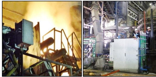
Figure 18. Lindarc™ receiver and control cabinet
