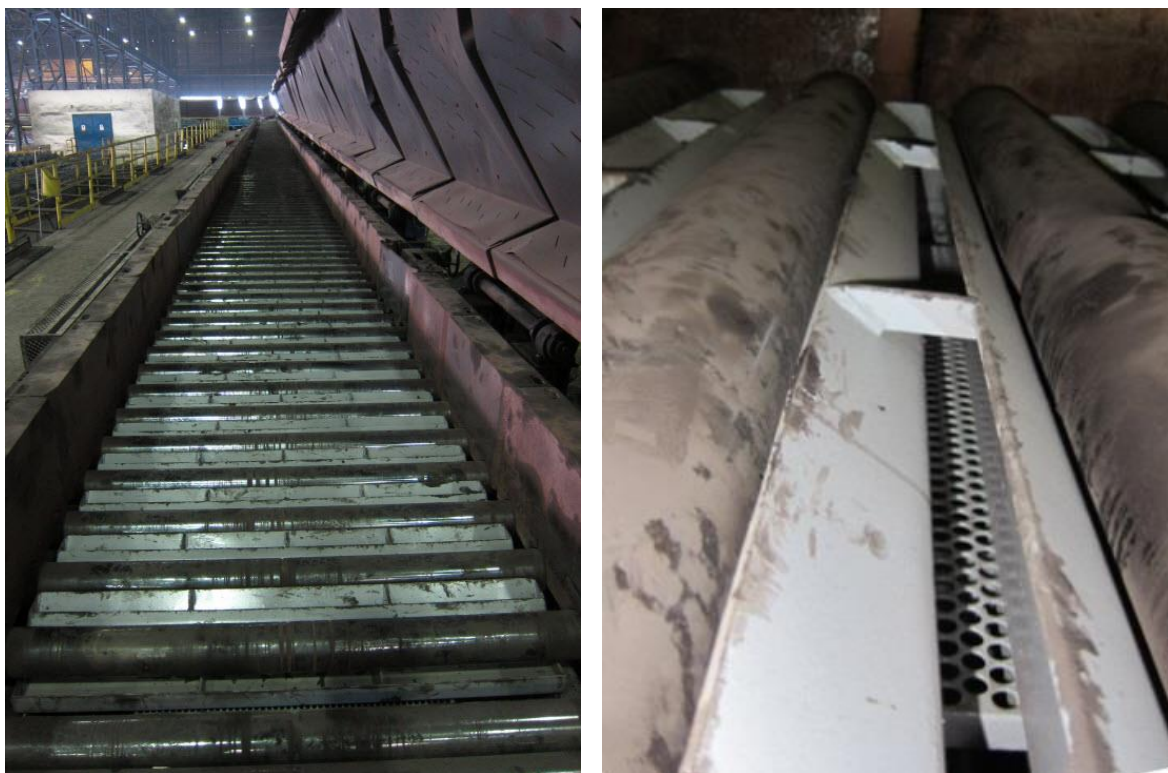
Figure 5. New conveyor section with angled nozzles and Optimesh system.
