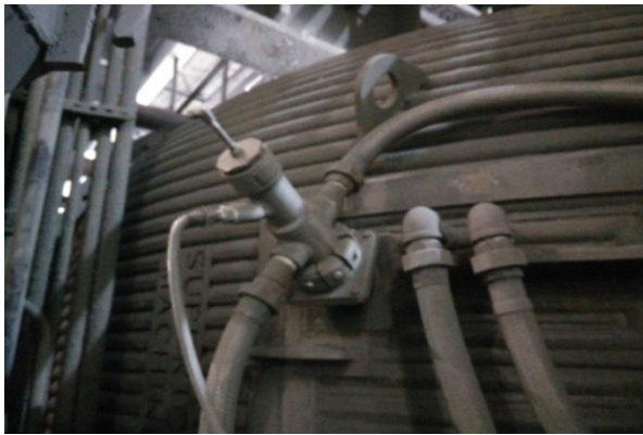
Figure 2: Down-stream Probe Location at SDI
